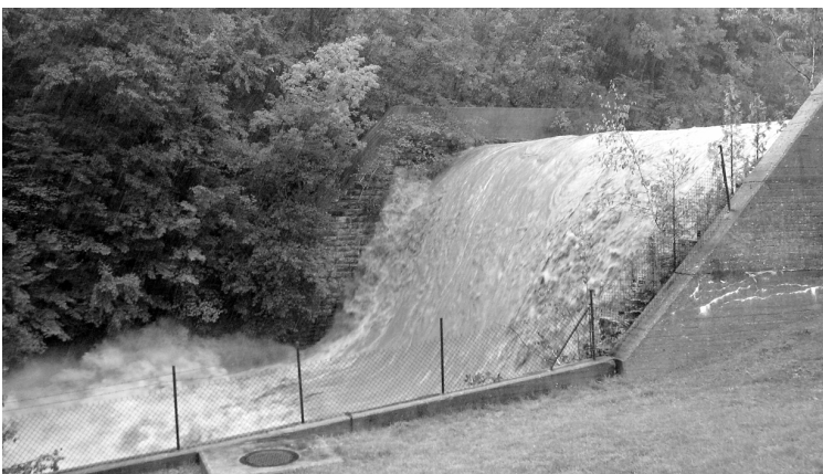
Eclipse Mill dam during tropical storm Irene. Photo by Judy Grinnell.
